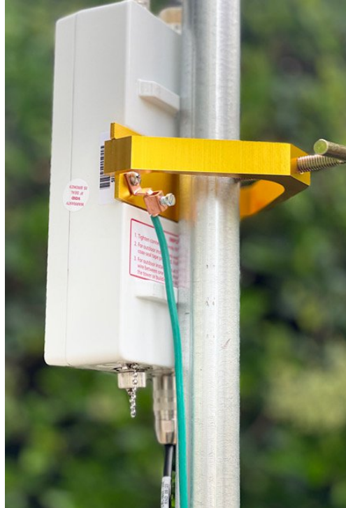
Figure 3.3 - pulsAR radio mounted on a pole
